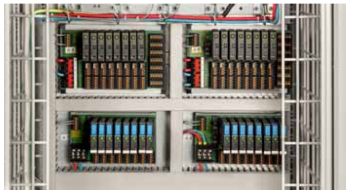
Power distribution systems SVS for ESX10-S and ESS20
