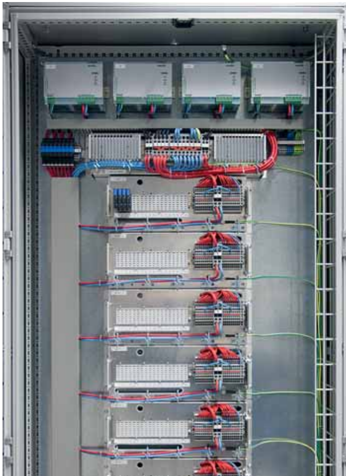
control cabinet SBG T018
