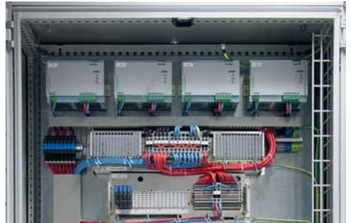
power supplies, diode de-coupling and protection
