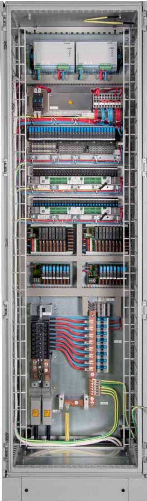
Demo control cabinet T029
